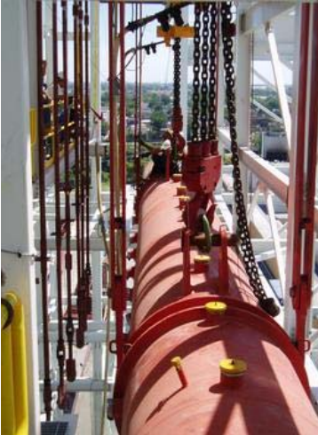
Once inside the structure, the drum is lowered on to its final mounting straps
